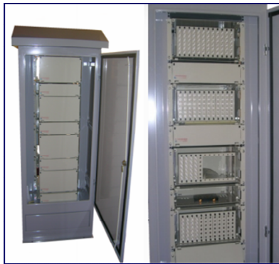
Outdoor Fiber Distribution Cabinet
